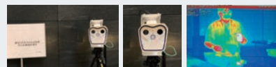
Install thermal cameras at entry / exit gates. Check the temperature of visitors.
